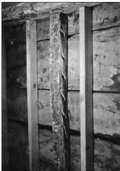
Figure 5. Post on west wall of borning room which shows the drill holes to take the ladder of support for wattle and daub, the earliest 17 th c. form of wall construction.
